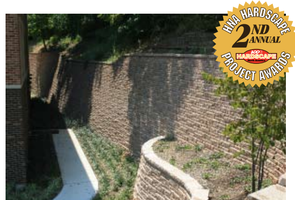
Terra Structures' award winning retaining wall at the Knollwood Military Retirement Residence in Washington, D.C.
