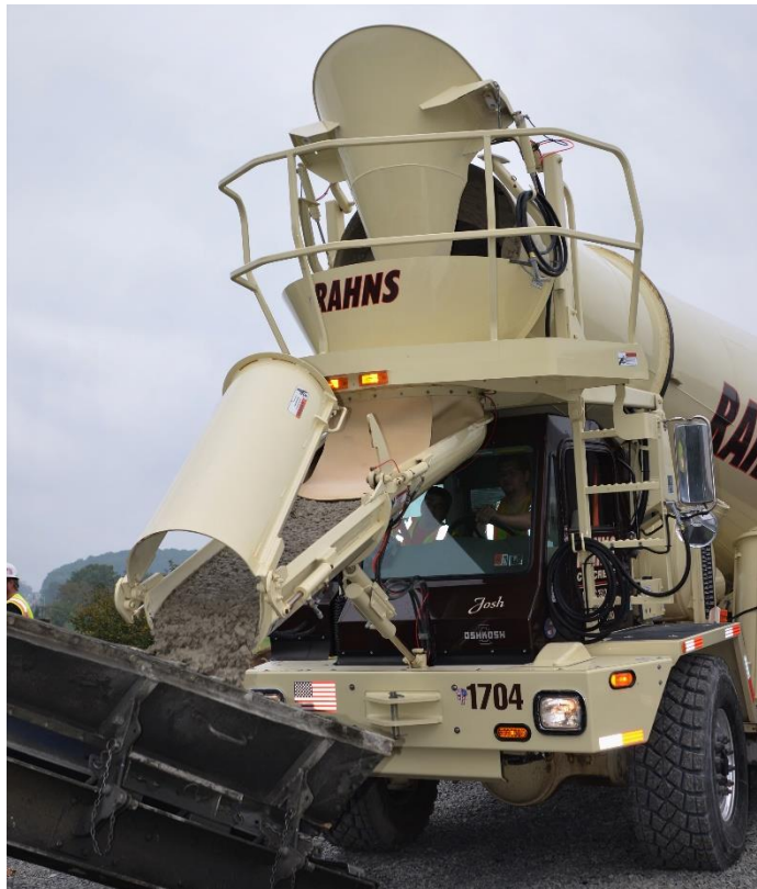
Pictured: A top-of-the-line RAHNS concrete truck in action on a job site.
